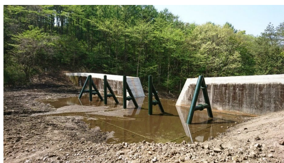
Photo Up to full-sediment level: Nagaigawa Sabo Dam (MLIT Tone River System Sabo Office)
