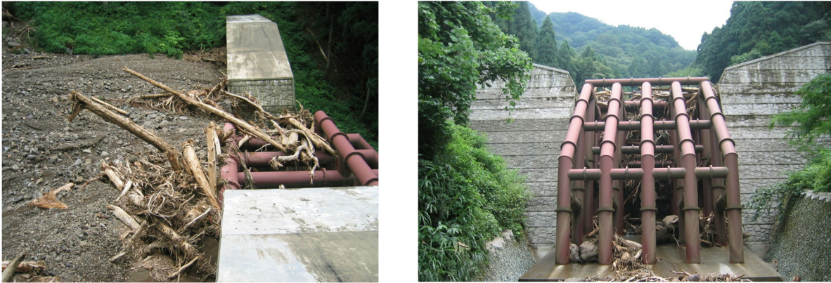
Photo 3: Hydraulically-consecutive Sabo dam that captures both debris flow and driftwood
