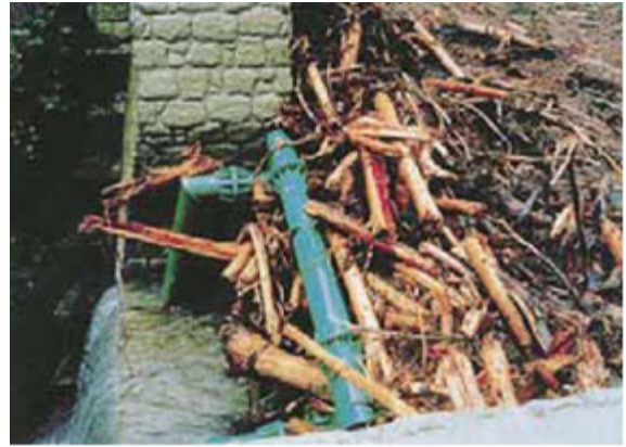
Photo 3 Driftwood captured by the driftwood entrapment structure of the secondary levee
