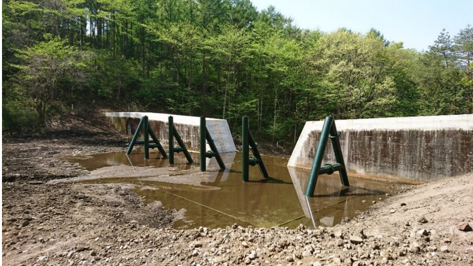
Photo 5: Up to full-sediment level: Nagaigawa Sabo Dam (MLIT Tone River System Sabo Office)
